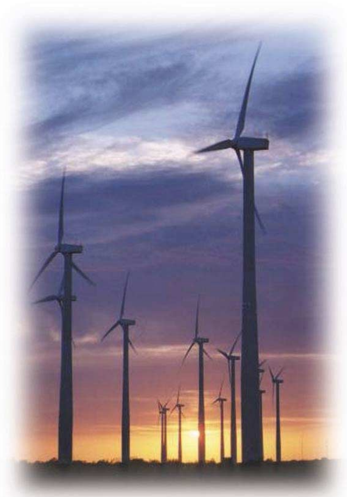
Moorhead Public Service, located 250 miles northwest of Minneapolis, chose an arctic model wind turbine generator from NEG Micon for its "Capture the Wind" green power program. (Photo courtesy of NEG Micon)
